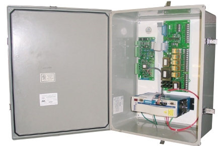
Operator Control Station
